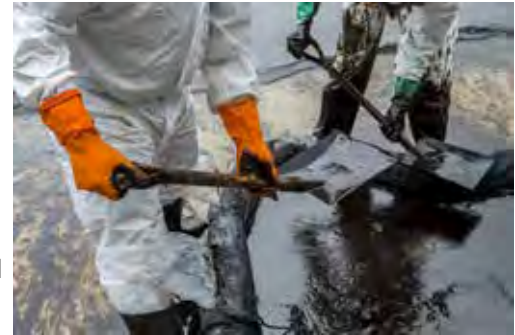
Clean up any bitumen spills.
